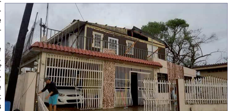
Jose and Kenysha's home devastated after the hurricane. (Photo courtesy of Jose and Kenysha Melendez)
