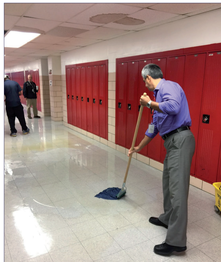
Mr. Perisic helps mop up the leaking water after heavy rains flooded the North Wing.
